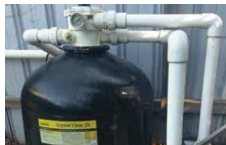
Doing annual maintenance on outdoor pumps, like the swimming pool pump shown here, can make it more energy efficient. Photo credit: Michael Coghlan
